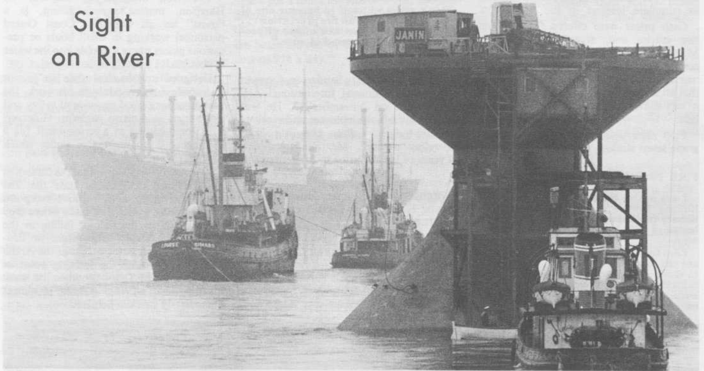
Site of the sinking of the Prince Shoal lighthouse caisson was a busy spot as the tugs jockeyed the giant structure into exact position.
